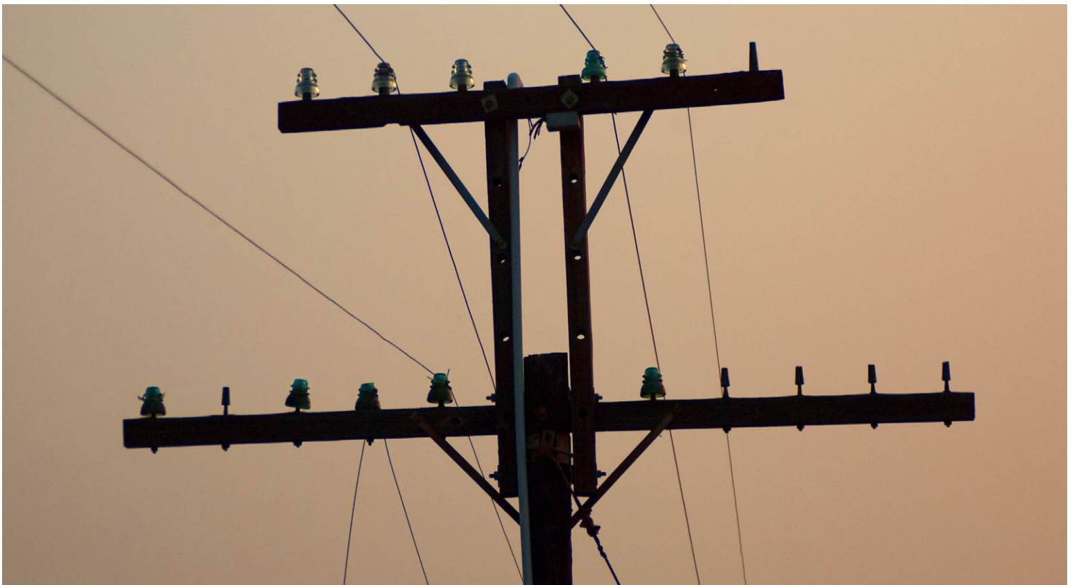
INSULATORS IN SMOKY SKIES AROUND NILES, CA DURING THE FIRES. (LOVE THE POLE EXTENSION!)
