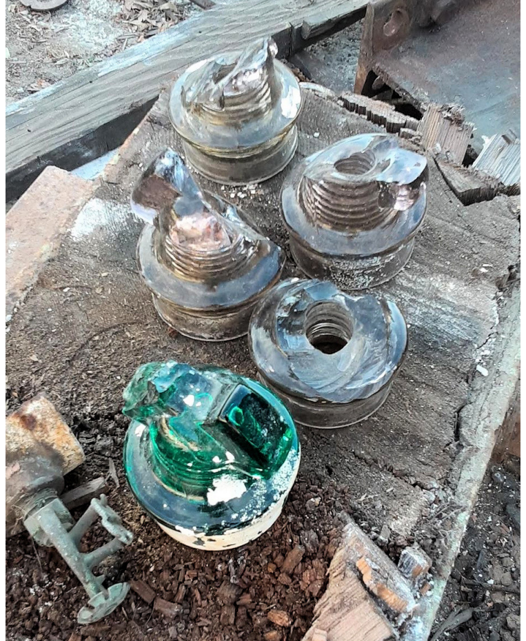
FIGURE 4 (LEFT & ABOVE): FOUR VIEWS OF THE FORMER MILL SITE. IN THE LOWER LEFT PHOTO, NOTE THE PINS AND INSULATORS ARE STILL ATTACHED TO SOME OF THE STACKED BEAMS
