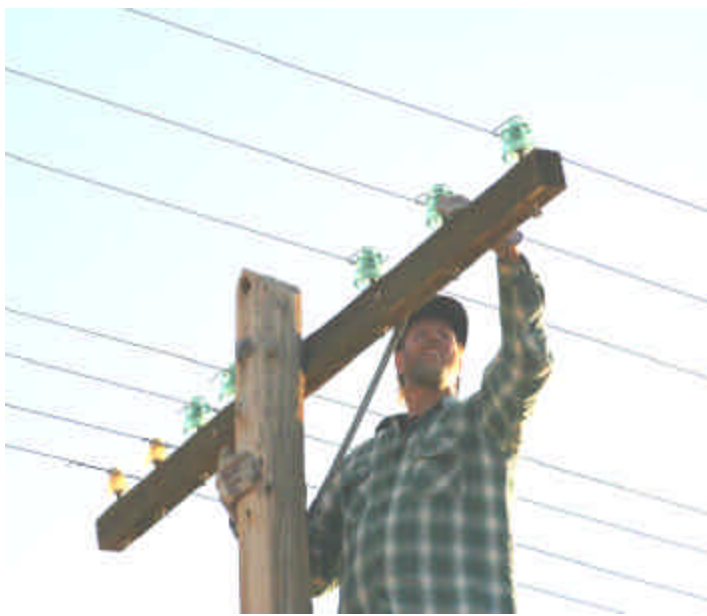
Roger Nagel examining one of the thousands of McLaughlin insulators on this line. Many with nails and Glazers points.
