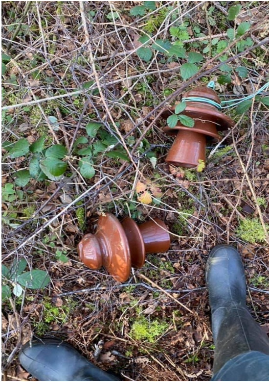
LEFT: PHOTO 3 – TWO P.5067S AFTER BEING RESCUED FROM THE POLE.
