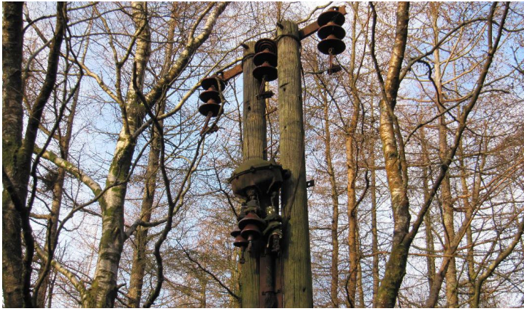
ABOVE: PHOTOS 9&10 – TYPICAL SWEPCO. TERMINAL POLE & ALEX RICE HOLDING THE THIRD UMBRELLA FROM THE FALLEN POLE, FOUND LYING NEAR THE POLE BASE.
